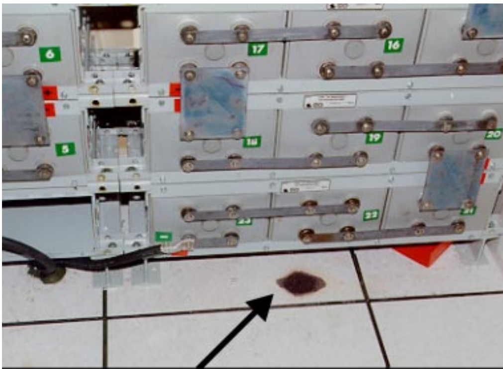
Figure 7.1. Signs of Electrolyte Leakage From a VRLA Battery.
